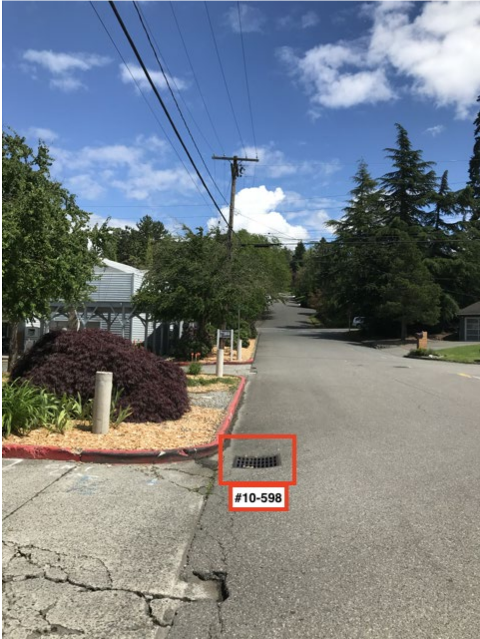
Facing E on the north side of SE 34th St, catch basin #10-598 in foreground.
