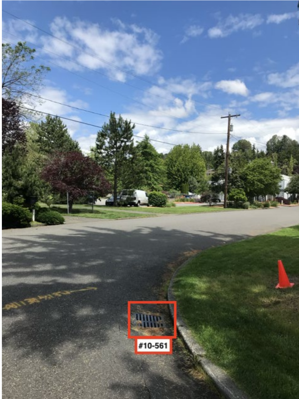
Facing NE, catch basin #10-561 in foreground (catch basin located on the southeast corner of the intersection of 77th Ave SE and SE 34th St).
