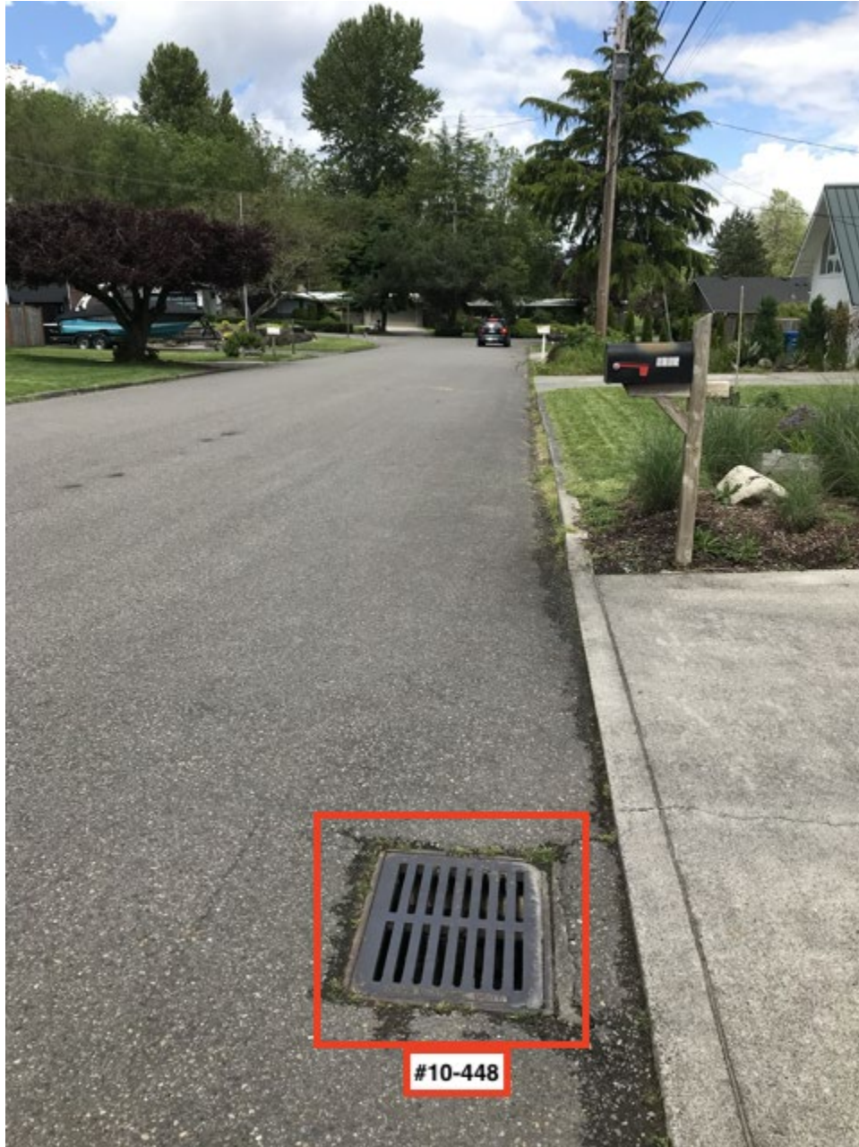
Facing N on the east side of 77th Ave SE, catch basin #10-448 in foreground.
